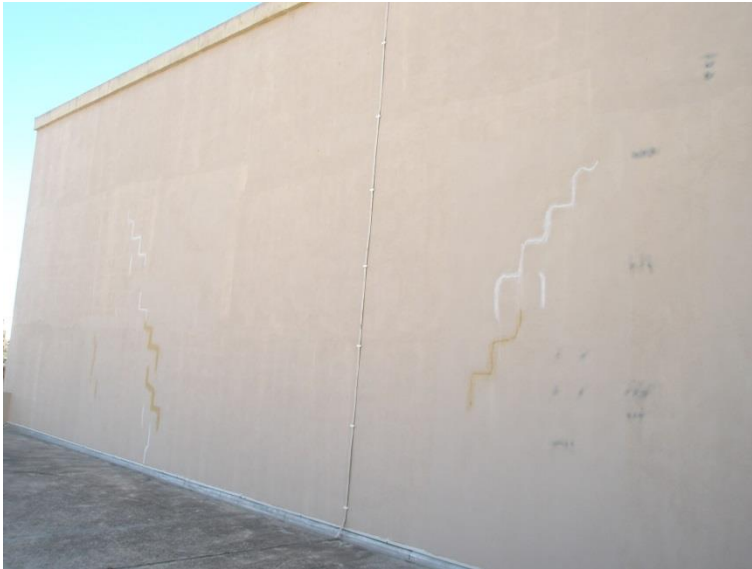
Figure 5 cracking in brickwork around plant room D1.3
